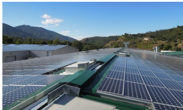
861 kW-Anlage La Gravona in Tavaco, Korsika
